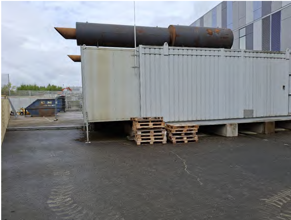
Photo 9 – Looking west toward existing generator (eastern most generator)
