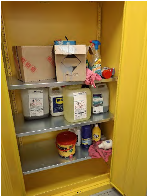
Photo 12- Inside COSHH cabinet, located within the Data Centre
