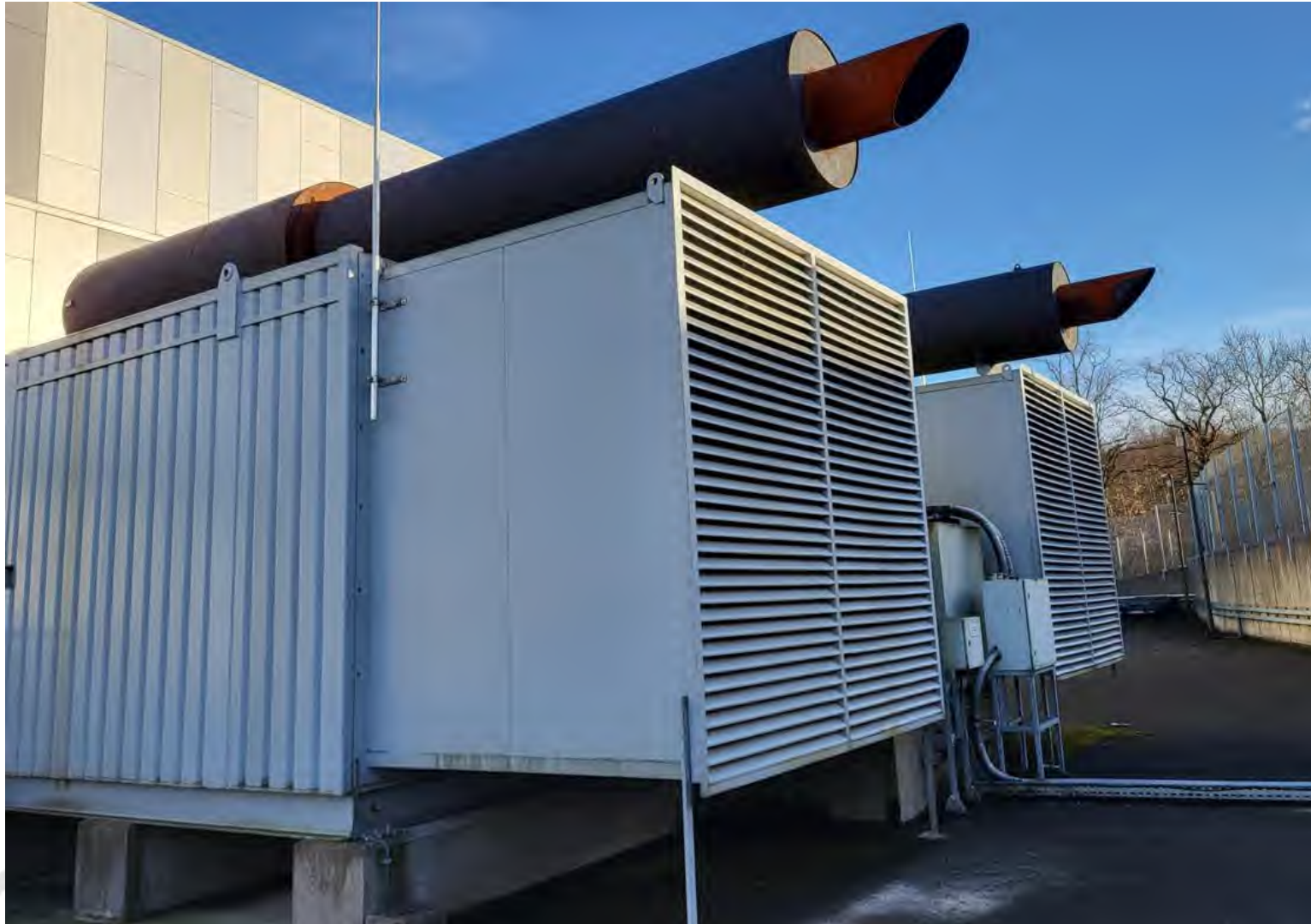
Figure A3.3 – Photograph of existing generator (facing outlet louvre and exhaust)
