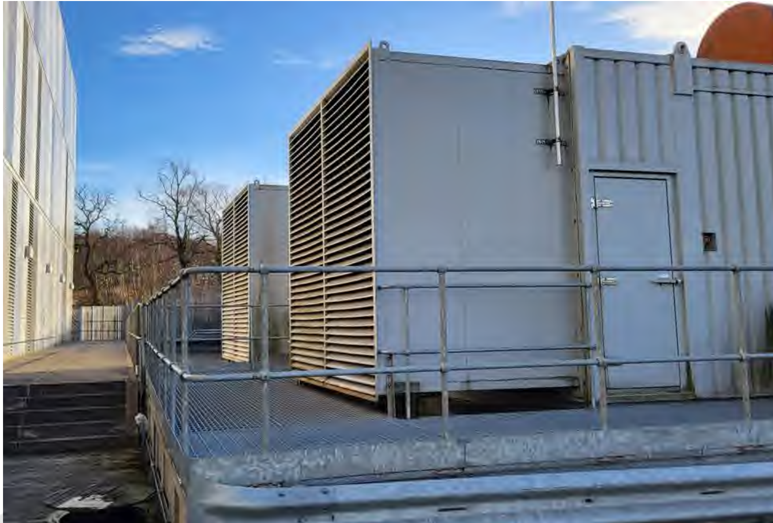
Figure A3.2 – Photograph of existing generator (facing inlet louvre)
