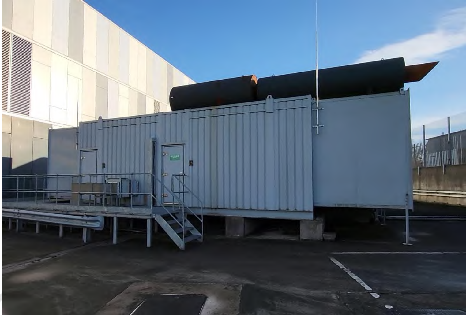
Figure A3.1 – Photograph of existing generator (side)
