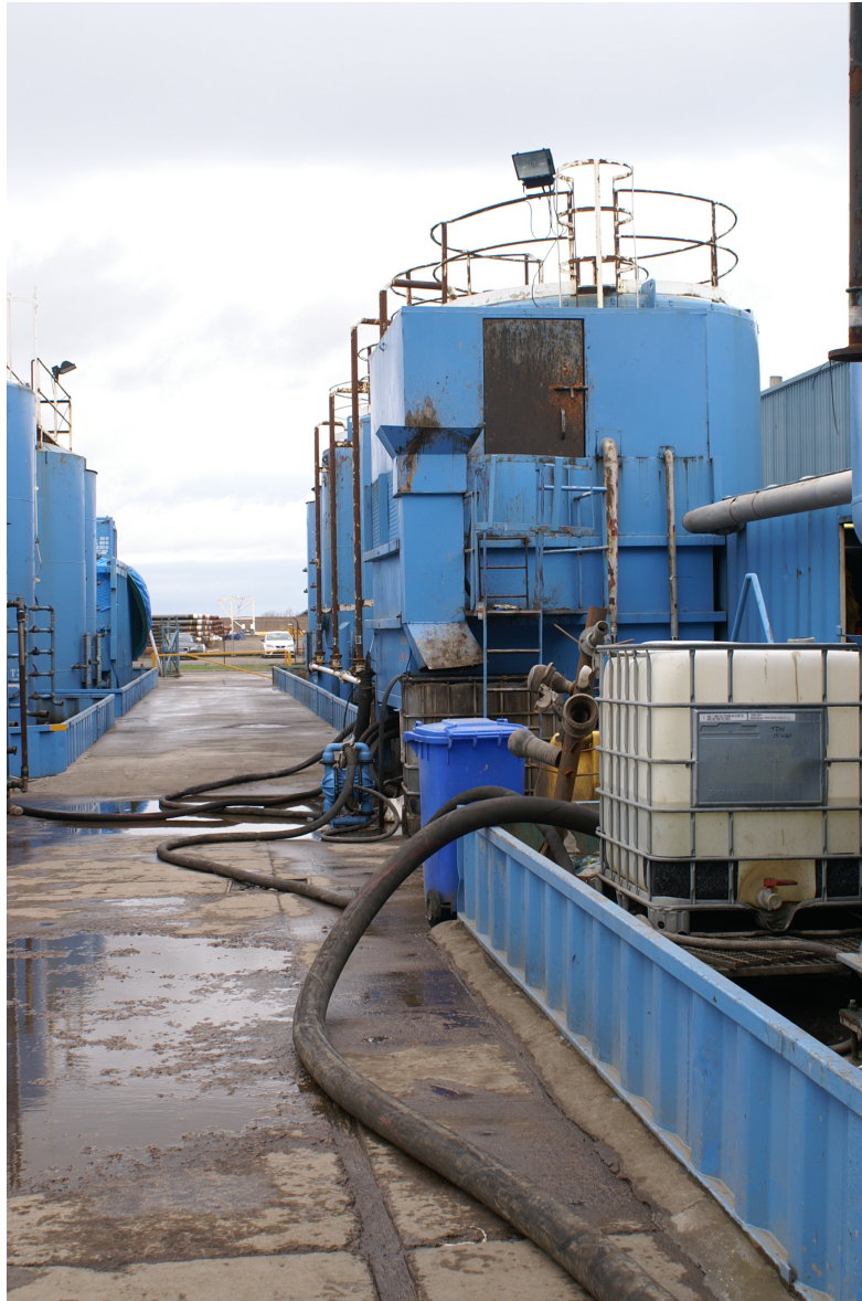
Photo 5 – Oil storage tanks on eastern site boundary with site secondary access gate in background.
