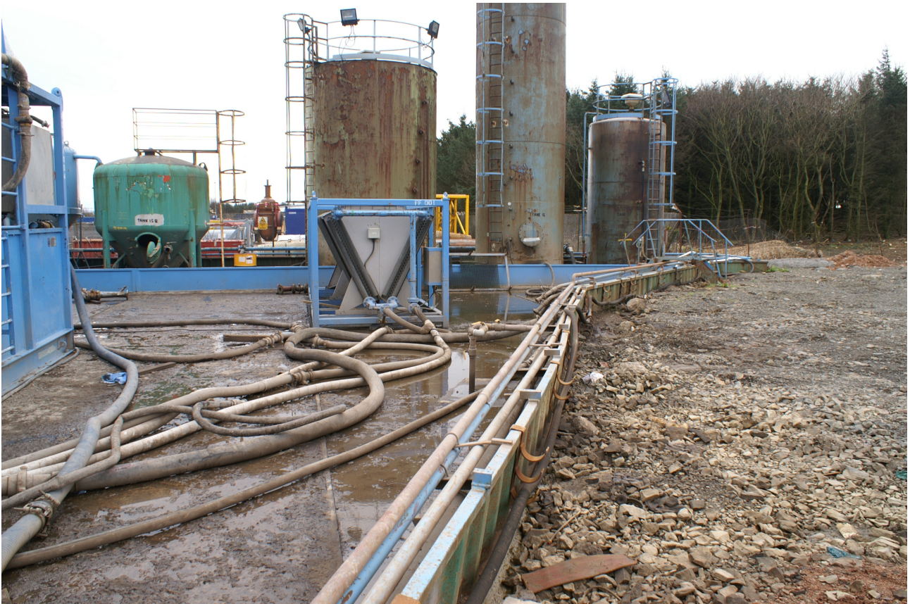
Photo 3 – Corrugated steel bund separating eastern operational area from unused hardstanding. Slight oil seepage noted during visit.
