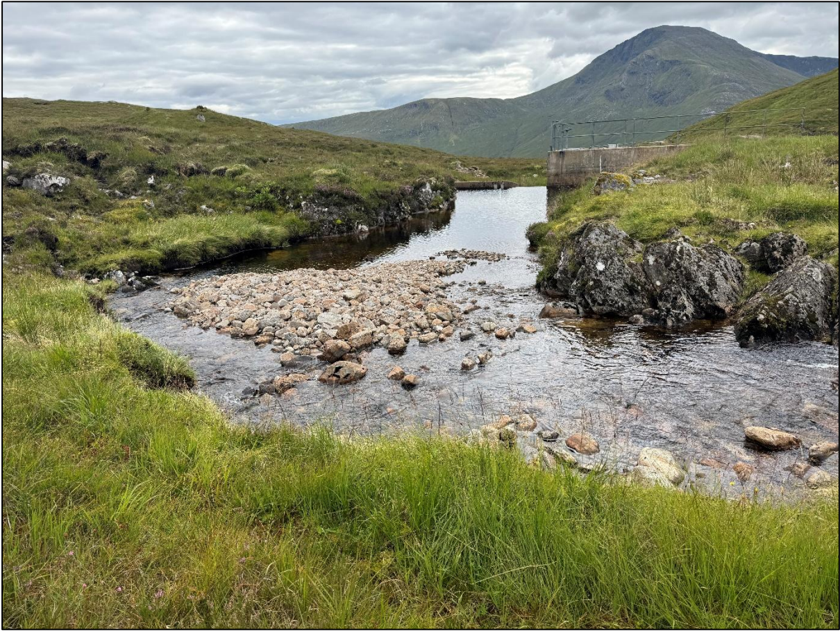
Figure 11. Alluvial sediment deposit located at the small hydropower intake structure on the Allt a Mheil at OS NGR NH 0465 0315.
