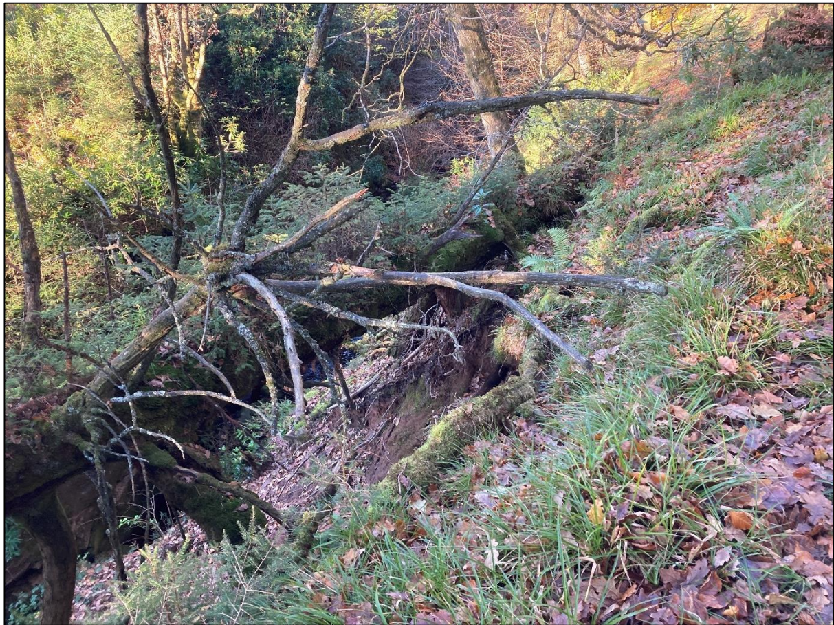
Figure 3.11. Landslip along riverbank
